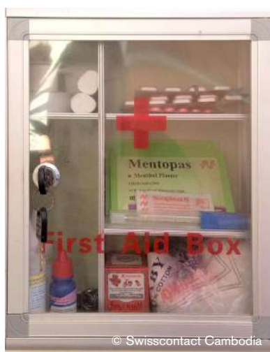
Figure 8, Installed first aid kit
